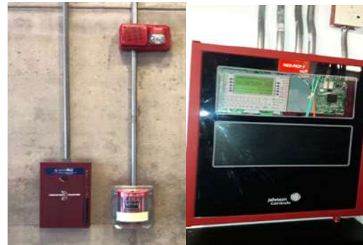
Figure 7. El Dorado Airport Fire Machine and FADS system, Terminal 1. Source: own.
