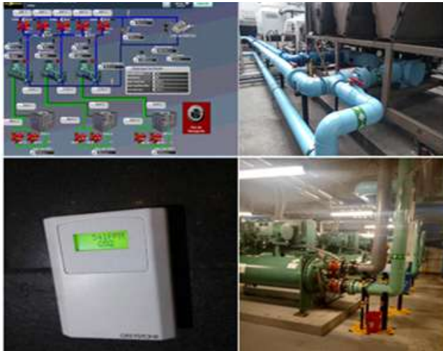
Figure 4. Integrated Air Conditioning Systems El Dorado International Airport. [22]
