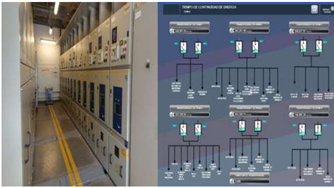
Figure 5. El Dorado Airport Electrical System Terminal 1. [36]
