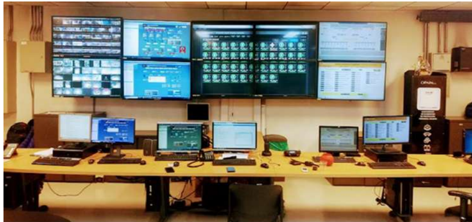
Figure 2. BMS system El Dorado International Airport. Source: own.
