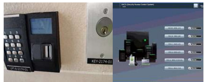
Figure 13. El Dorado Airport SACS system, Terminal 1. Source: own.
