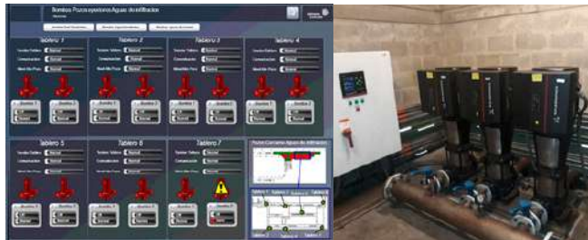
Figure 11. El Dorado Airport Plumbing System Terminal 1. [47]
