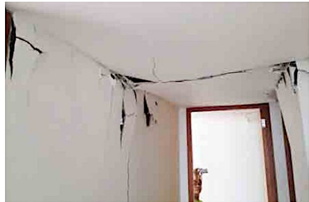
Figure 10. Cracks and fissures in dividing walls (Suárez, 2019).
