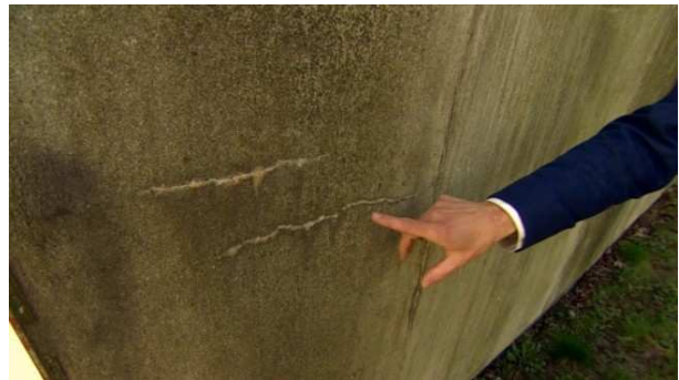
Figure 13. Cracked wall already repaired (Alvarez, 2017).
