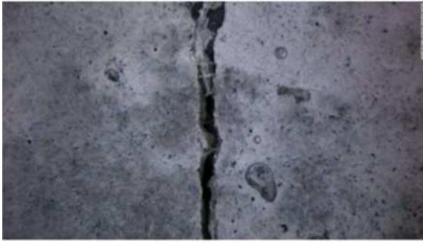
Figure 10. Concrete slab with freshly formed cracks (Alvarez, 2017).
