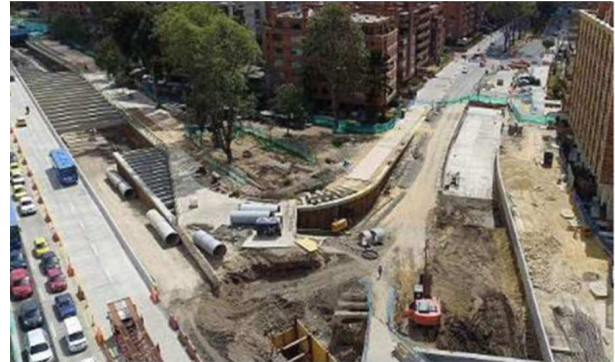
Figure 3. Unfinished works in Bogotá (Vernot, 2016).
