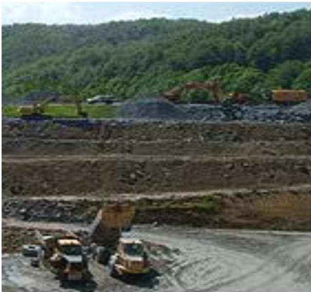
Figure 5. Unfinished works (Obras, 2017).
